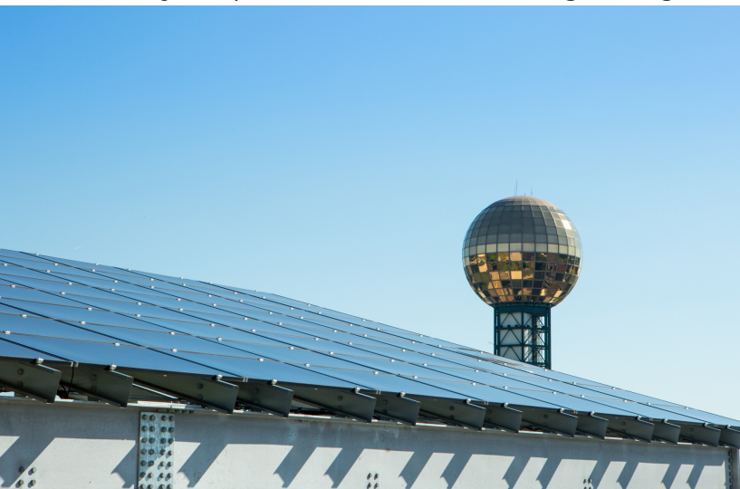
Solar array atop the 11th Street Parking Garage
